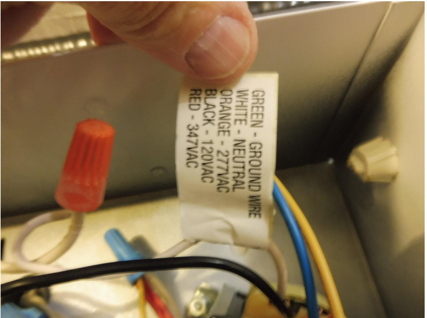
Photo 4: Tag on the input transformer showing the different input wiring.
