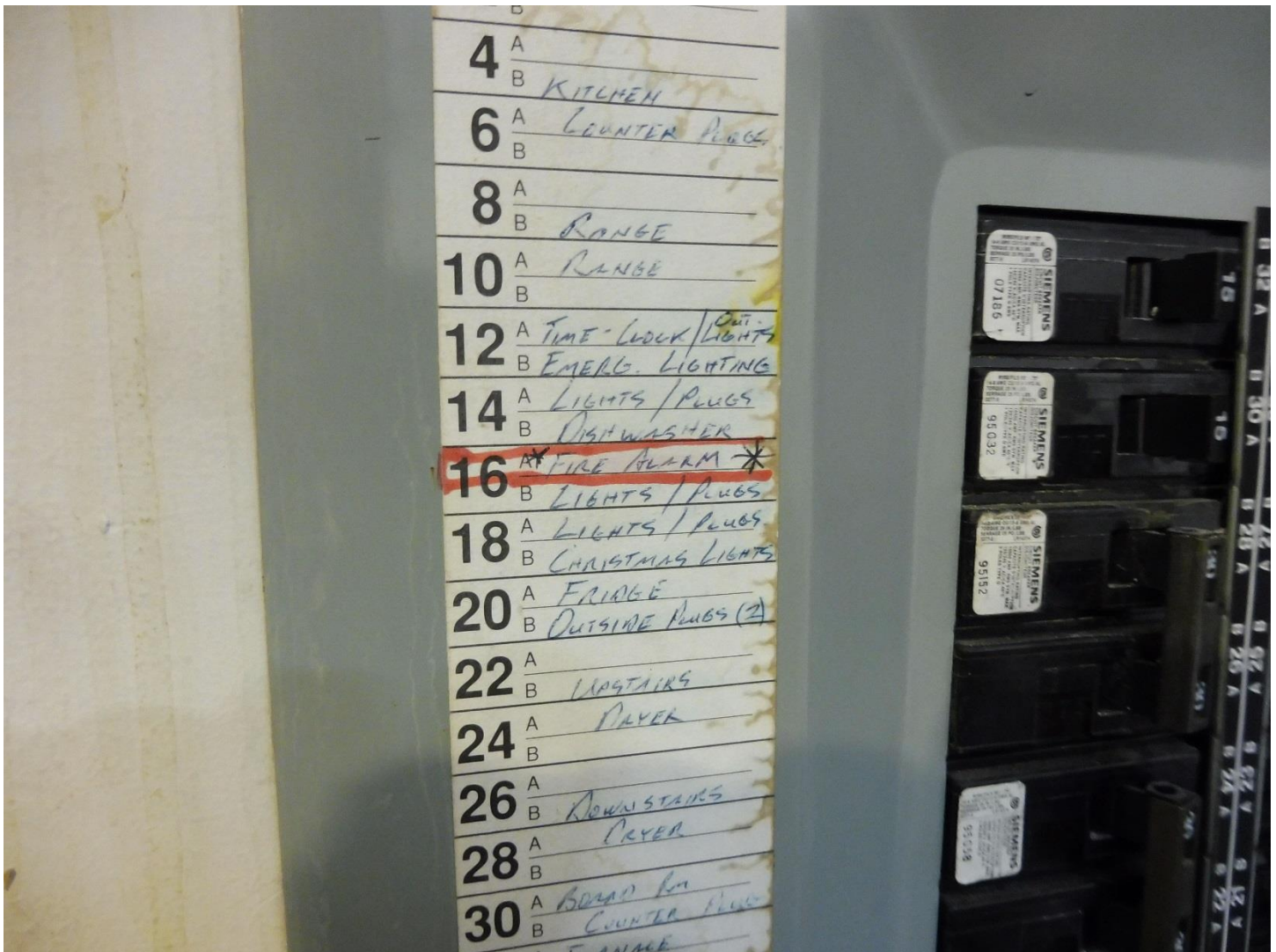
Photo 2: As noted on the panel directory circuit 12B supplies the emergency lighting pack.
