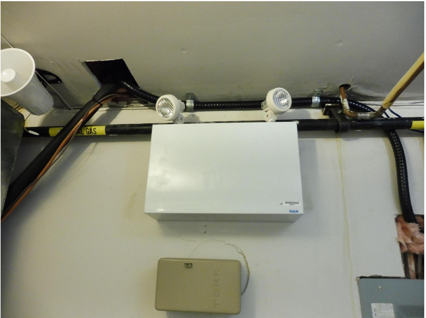
Photo 1: The emergency lighting pack is situated just to the right and above the electrical distribution panel that supplies it.
