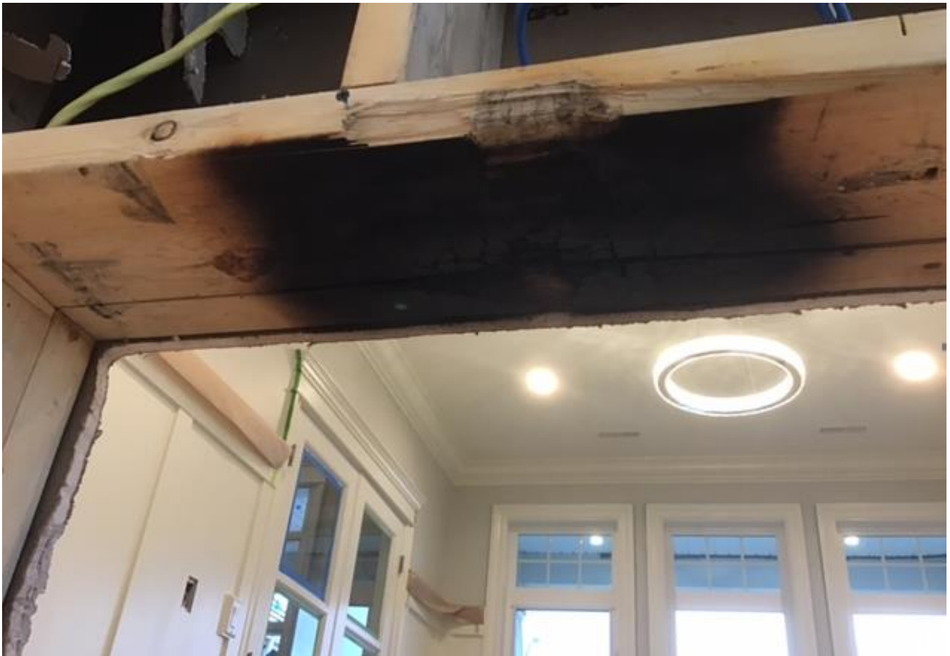
Photo 2: Damage to the wooden framing surrounding the fireplace location.
