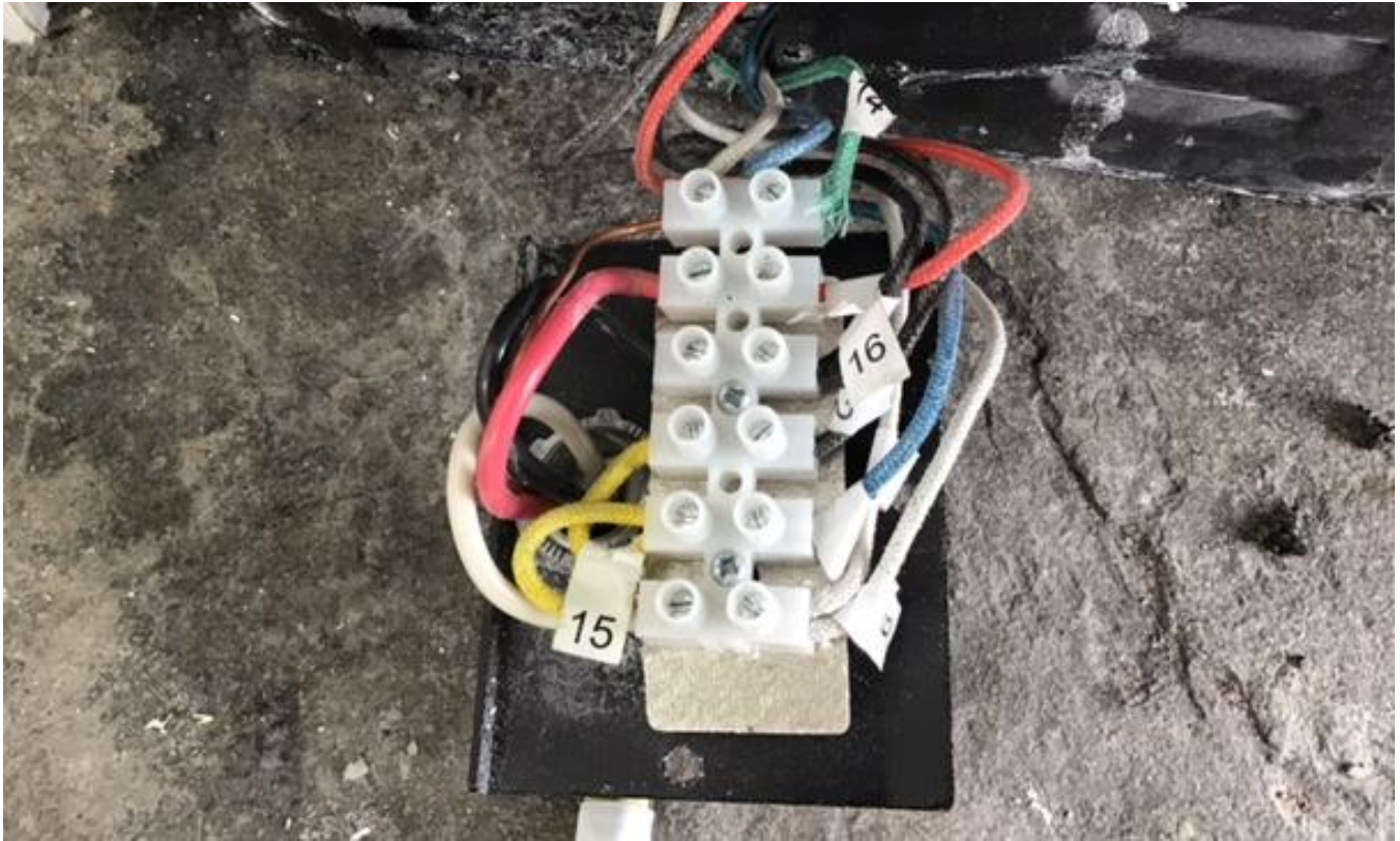
Photo 7: Yellow jumpers installed on fireplace terminal block.
