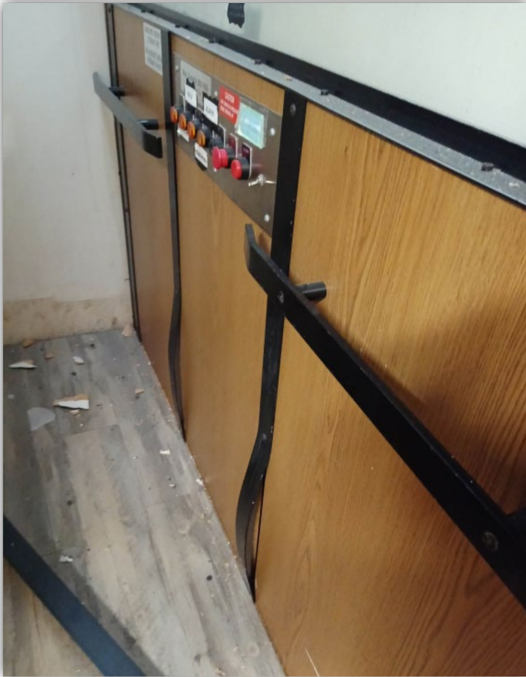
Photo 1 – Lift showing damage from drop into pit.
