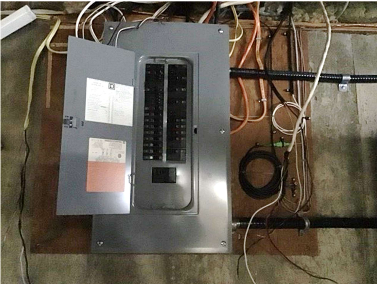
Main dwelling panel board, installed on basement level
