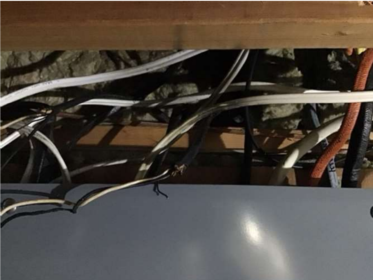
Burnt branch wiring cable insulation above panel board
