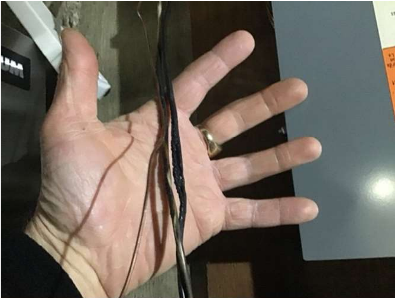
Burnt branch wiring conductor insulation
