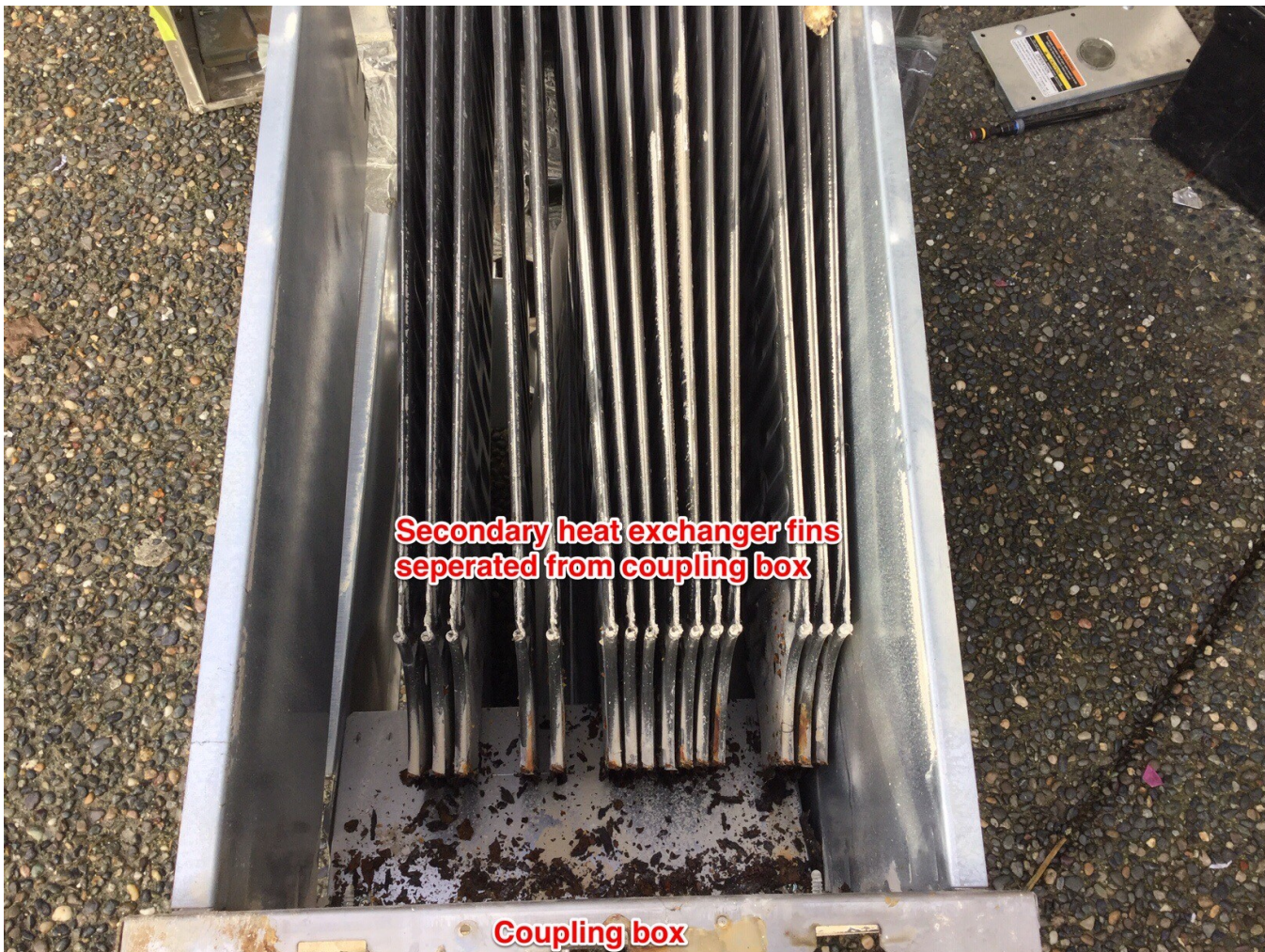
Image 3 – Heat exchanger removed from furnace and dismantled. End screws on the heat exchanger cabinet and secondary heat exchanger tubes had completely separated from the coupling box
