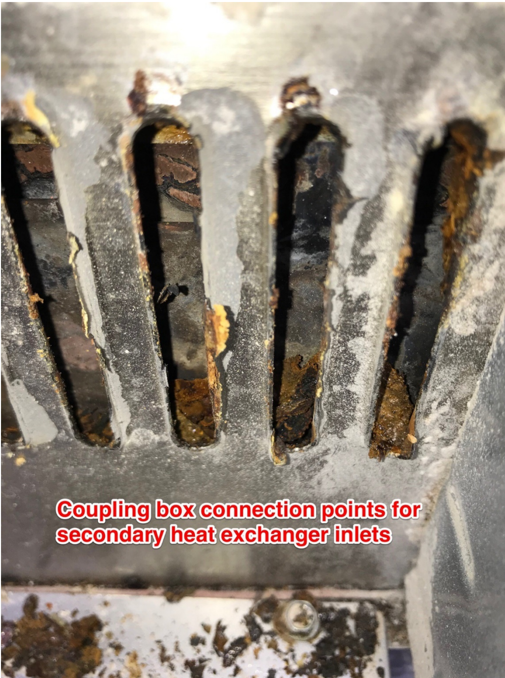
Image 7 - Secondary heat exchanger tube inlet connection points to the coupling box
