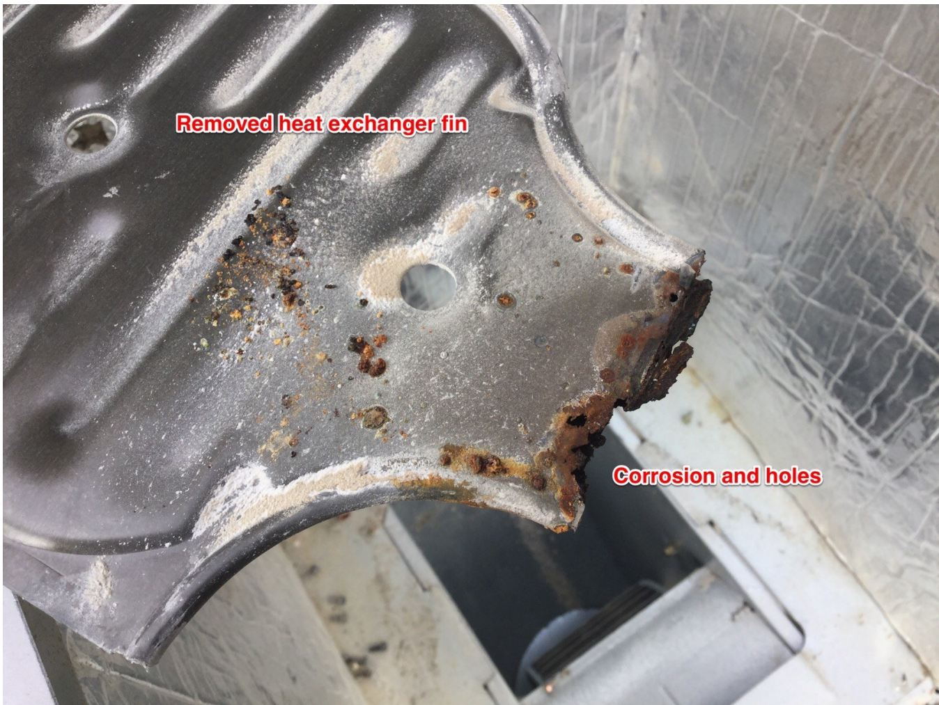
Image 5 - Secondary heat exchanger tube inlet
