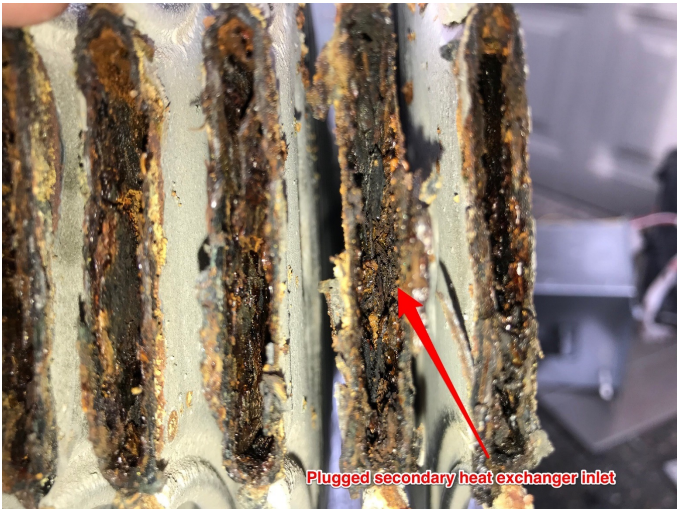
Image 6 - Secondary heat exchanger tube inlets
