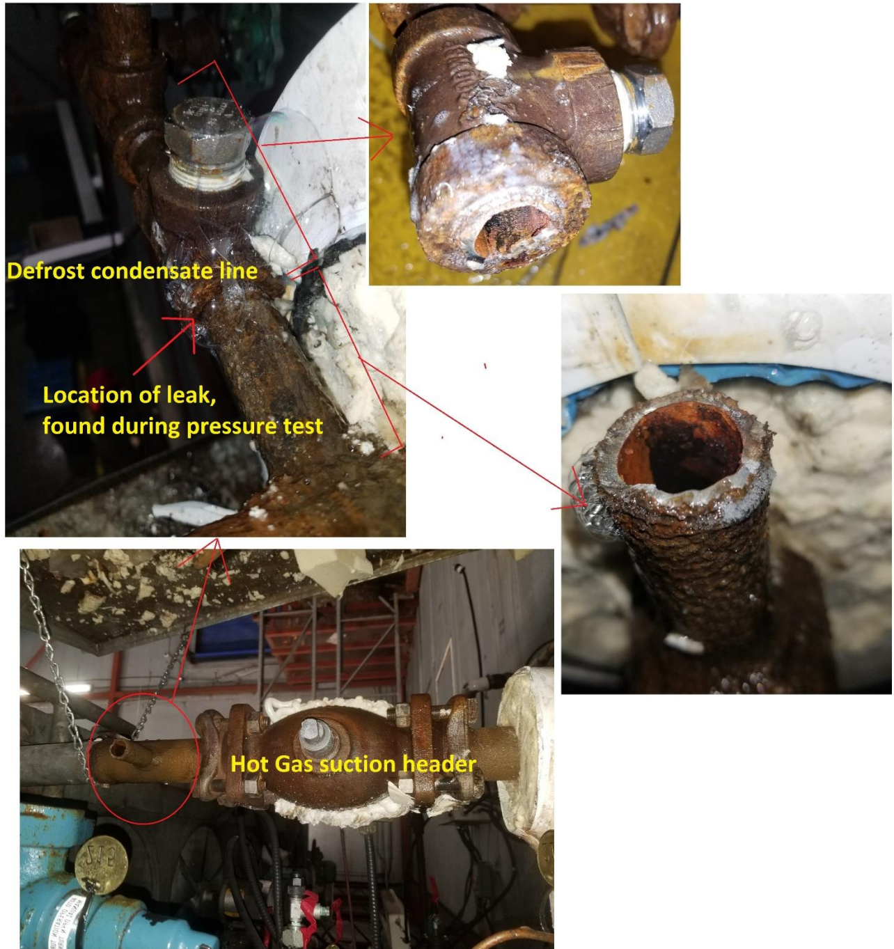
Fig. 3: Location of Leak (Image provided by repairing contractor)
