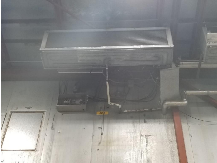
Fig. 1: Evaporator (Image provided by repairing contractor)
