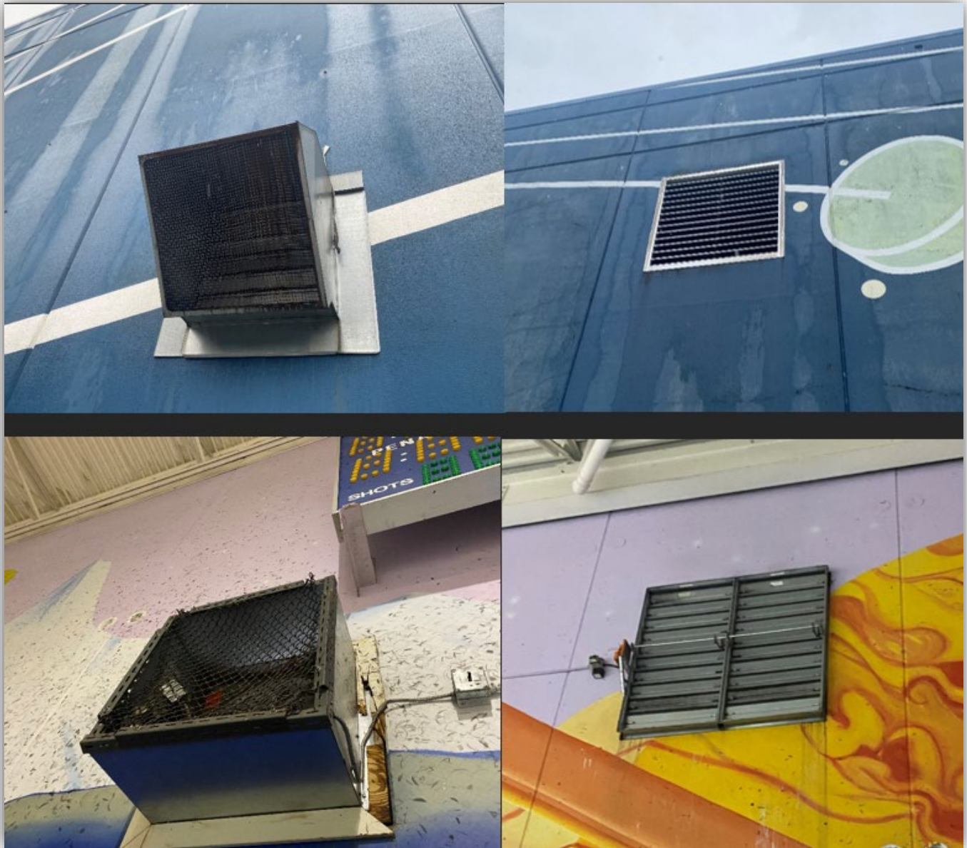
Image 7 – Left – The outdoor and indoor views of the rink 2 ventilation fan. Right – The outdoor and indoor view of the rink 2 louvered ventilation intake grate.
