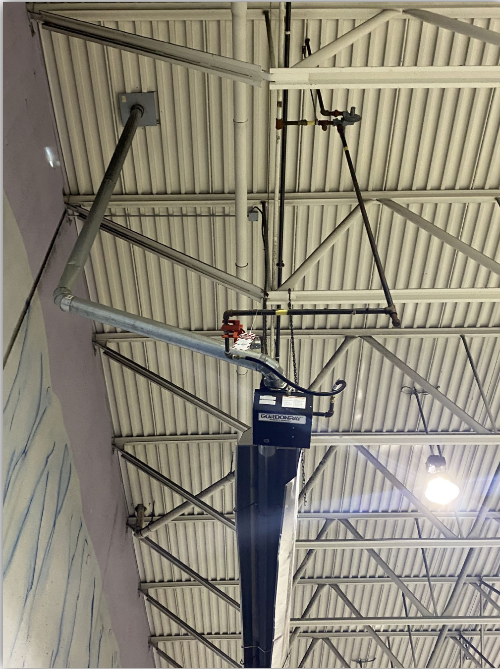
Image 3 – Air intake piping and burner unit for tube heater #1 on rink 2.
