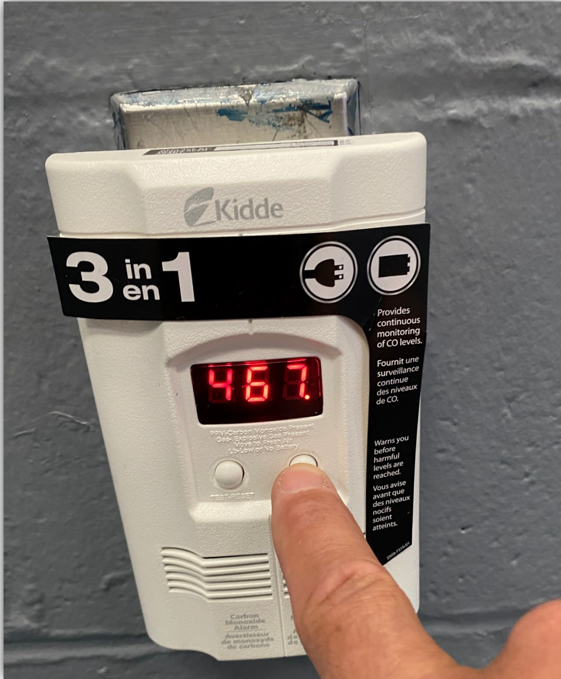
Image 6 – New CO detector installed in the building lobby showing a recall of a maximum reading of 467ppm.
