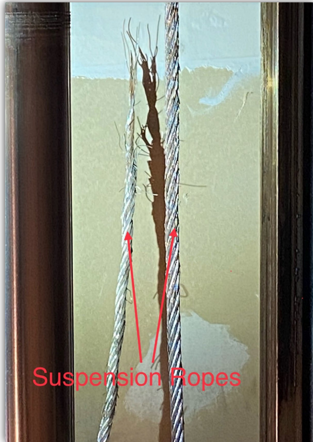
Image 3 - Severed suspension ropes.
