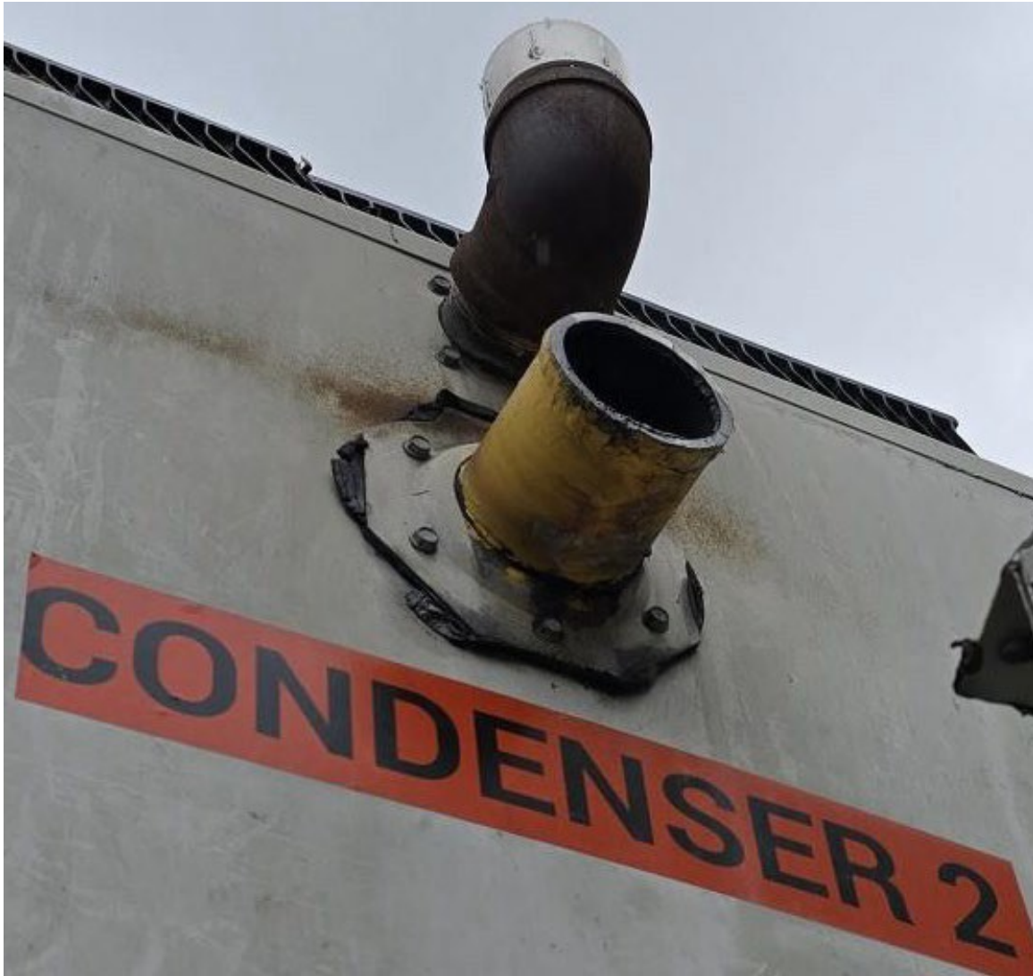
Image 3 - Ammonia Vapour Piping (yellow) after being completely cut.
