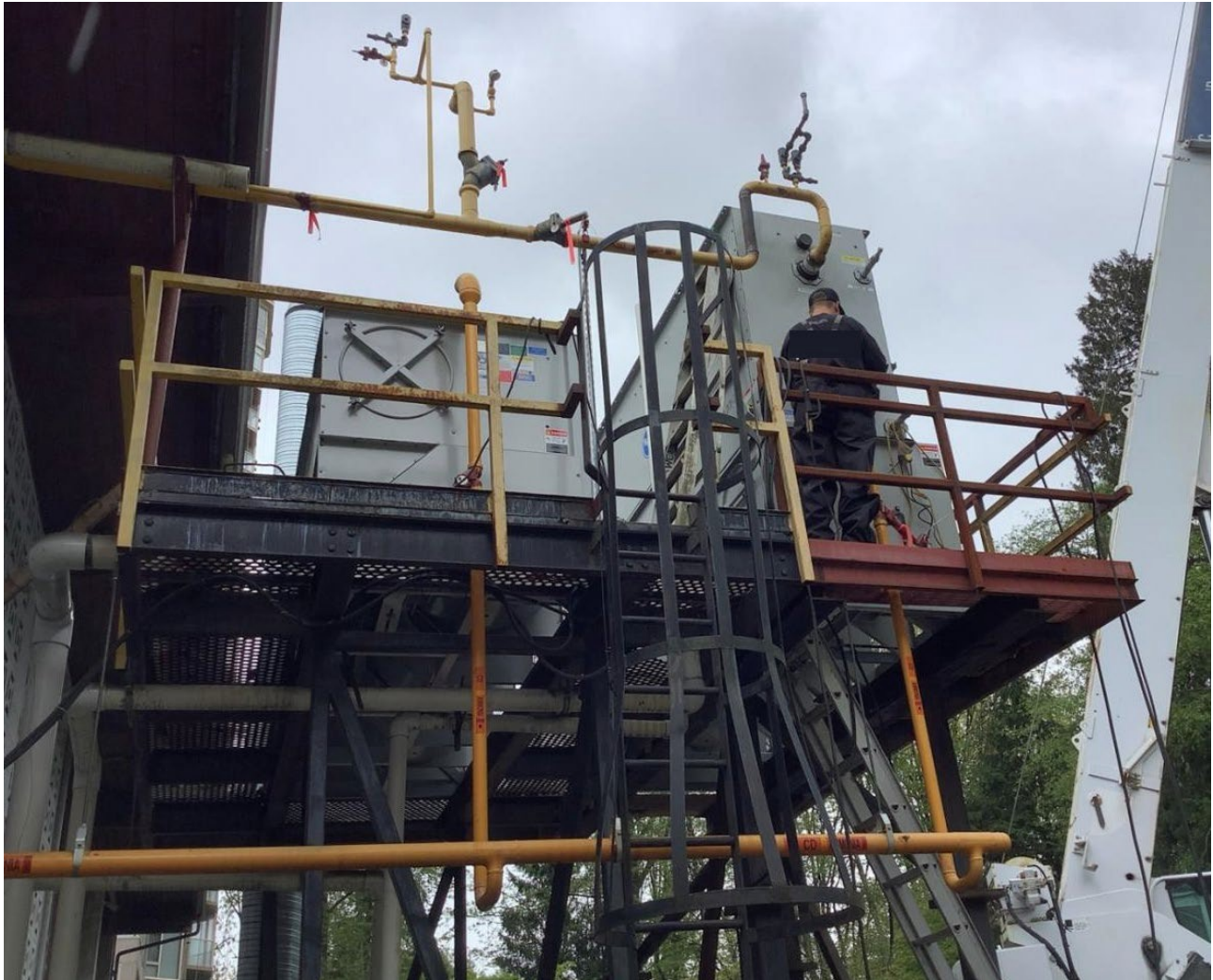
Image 1 - Ammonia condensers installed on the raised metal structure with connected yellow ammonia piping.
