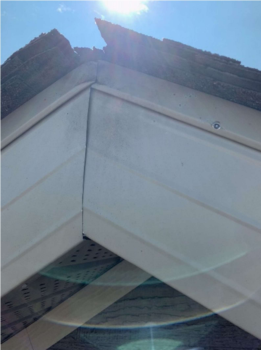
Image 4 - Roof peak where lightning hit the house
