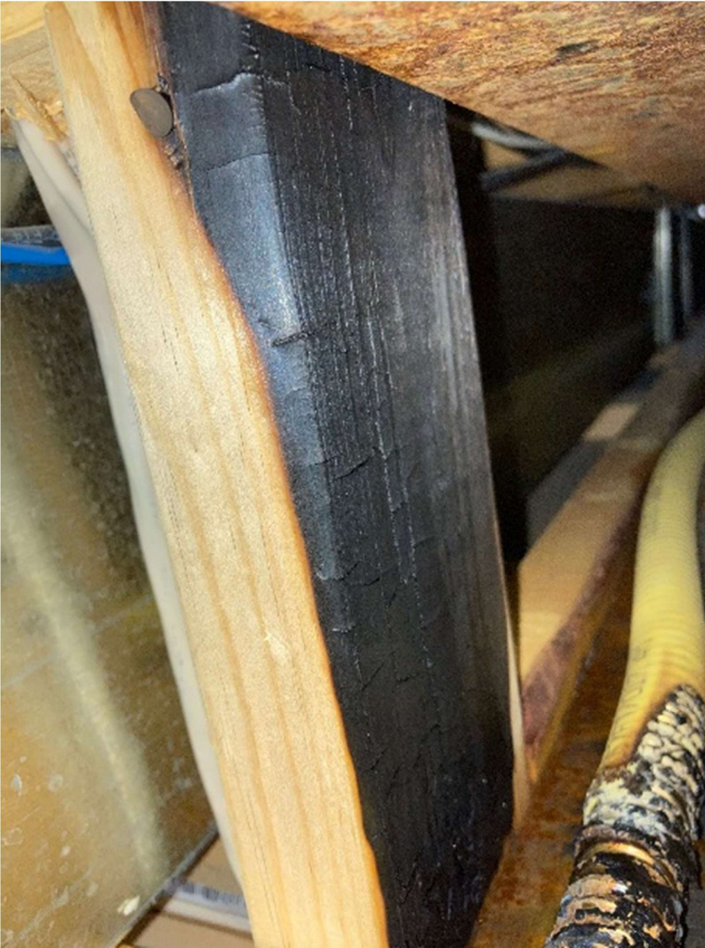
Image 3 - Fire damage to wood framing next to hole in CSST
