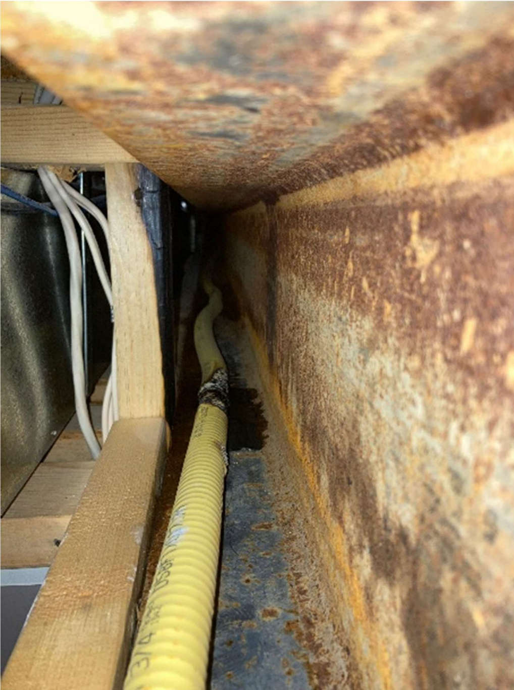
Image 1 - CSST run along structural steel beam.
