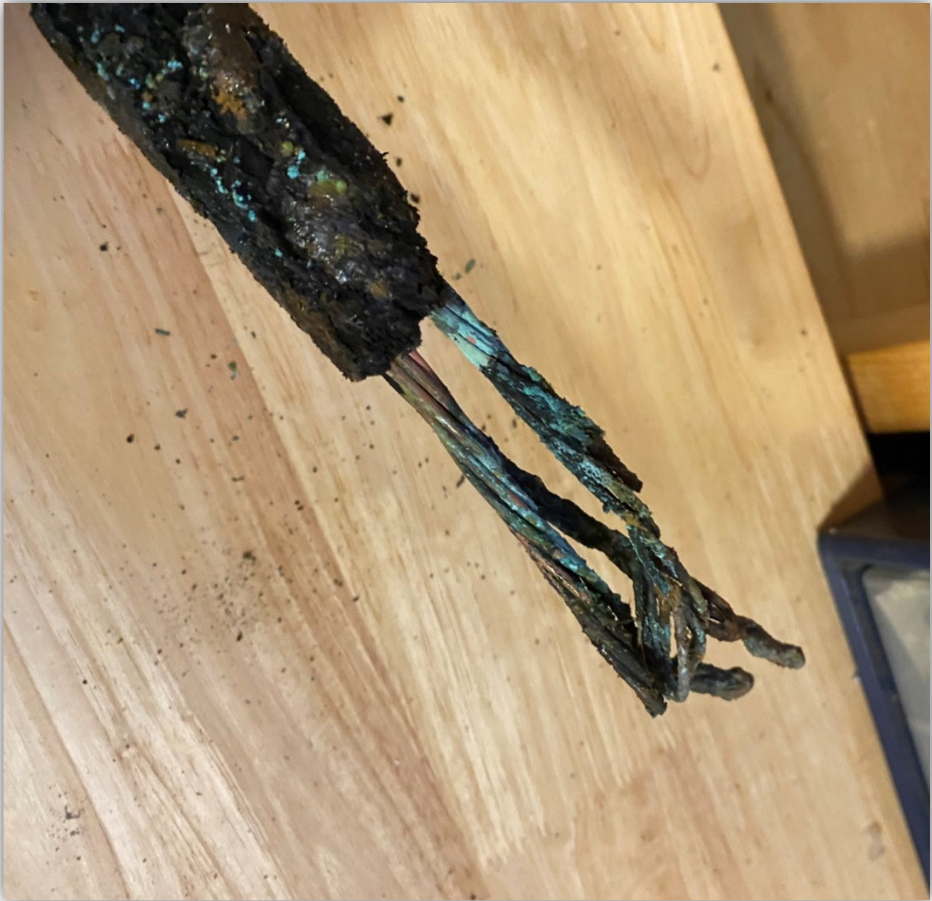
Image 8 - Insulation failed, bare consumer service conductors.
