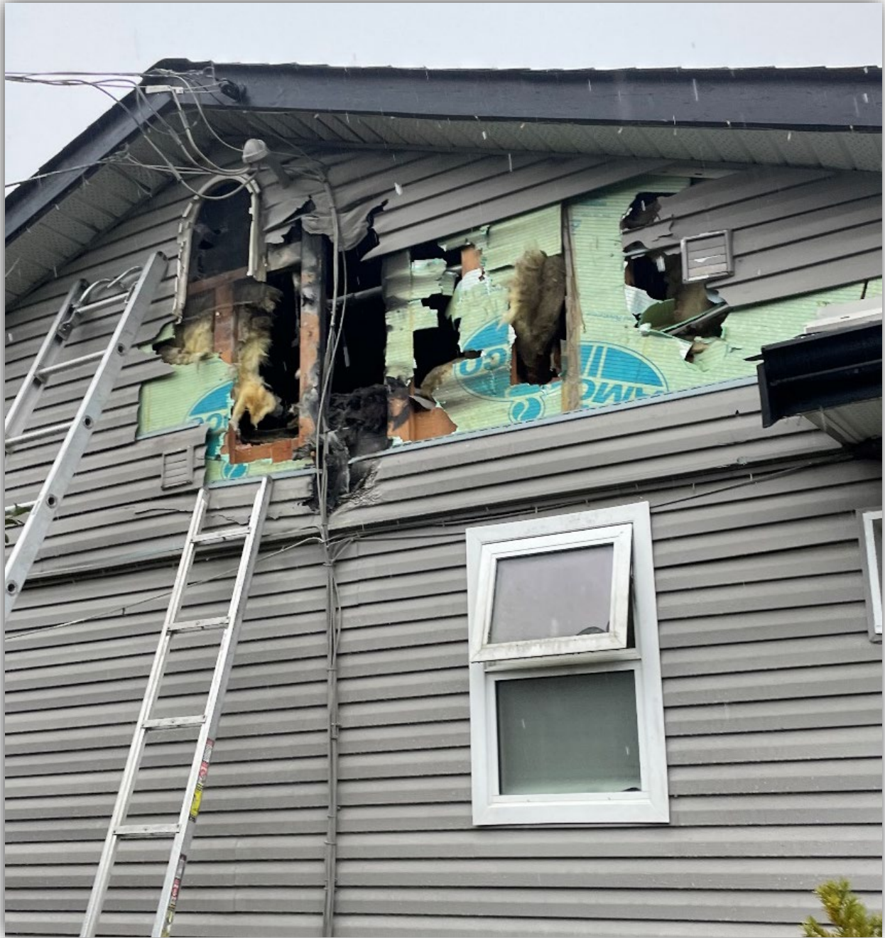
Image 1 - Fire in the attic and on exterior of the single-family dwelling.
