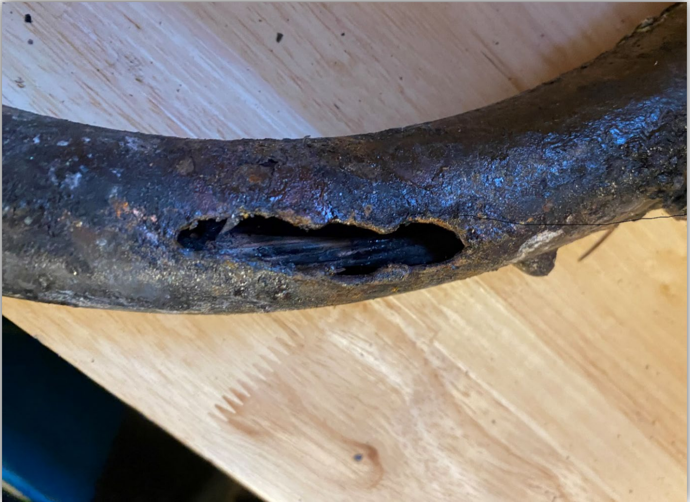
Image 3 - Bare conductors in the service conduit. The service conductor arced through the metallic service conduit in the attic.
