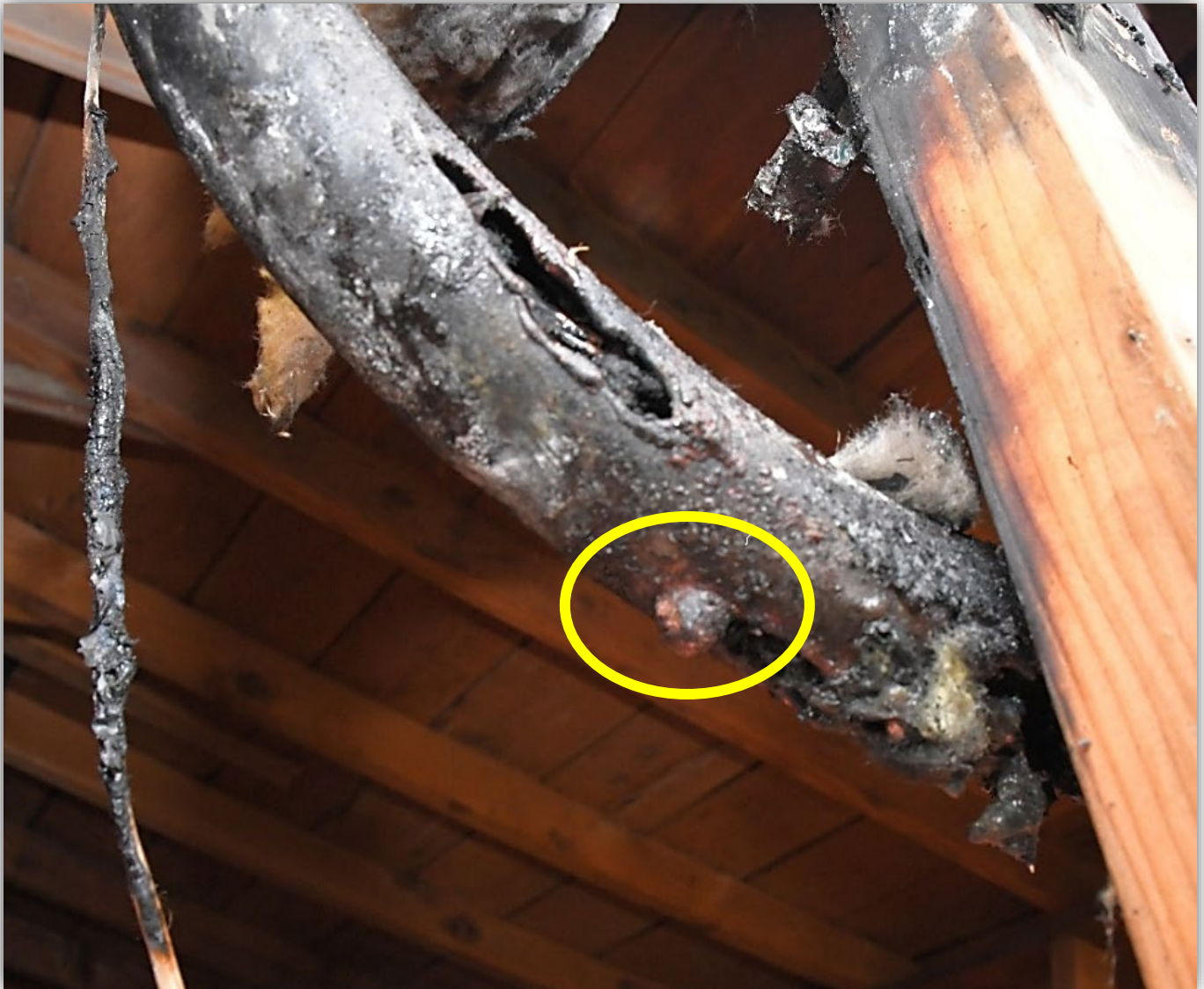
Image 4 - Bare conductors in the service conduit. The service conductor arced through the metallic service conduit in the attic. [Circle] Molten drip.
