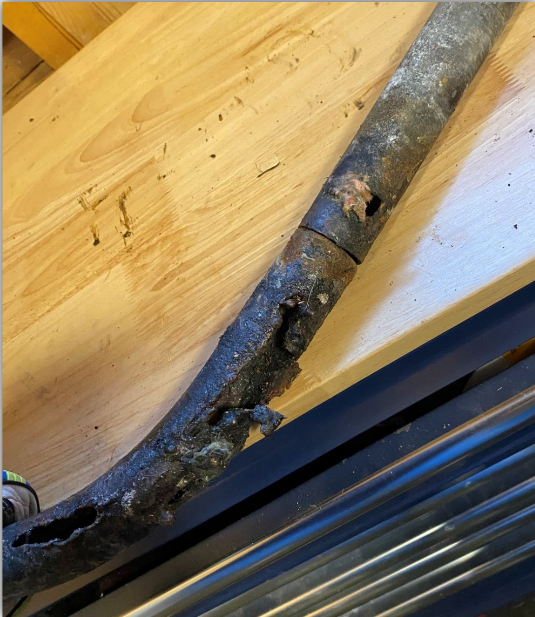
Image 7 - No evidence of a coupling, possible tampering.
