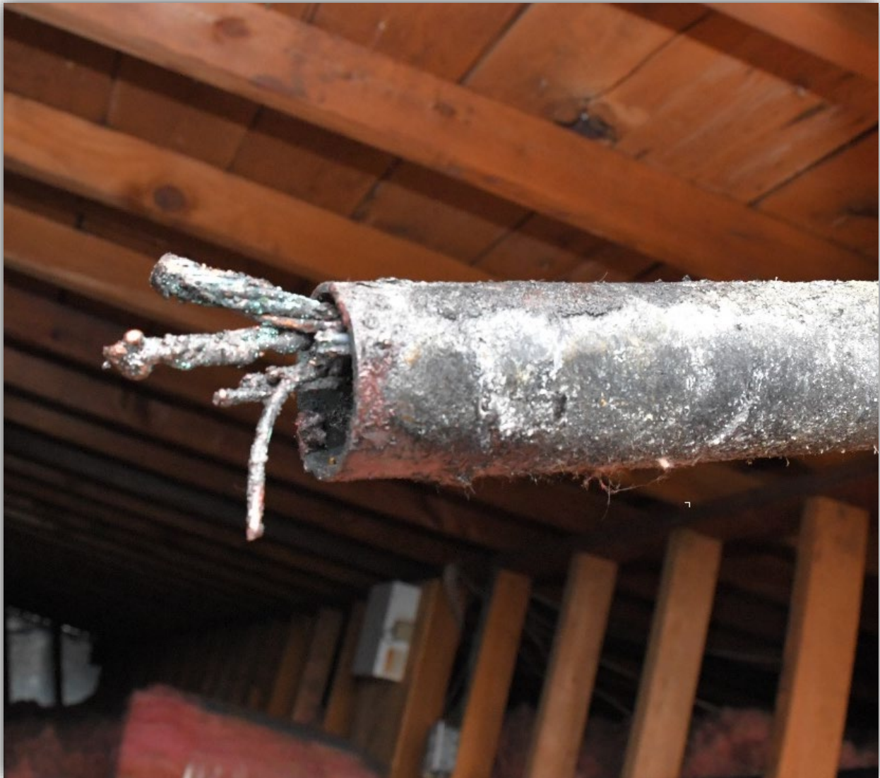
Image 5 - The service conductors with their insulation burned off and arcing at the ends of the conductors.
