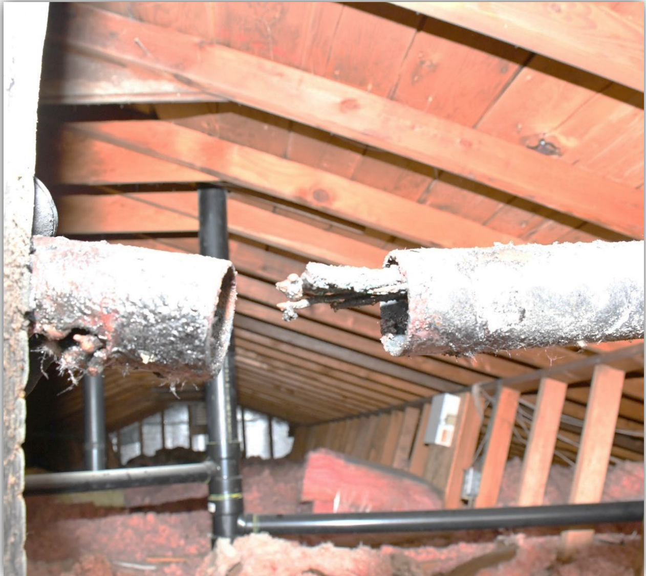
Image 6 – No evidence of a service conduit coupling.
