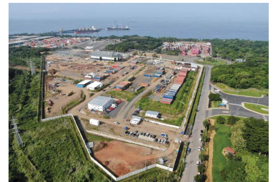
Our Energía del Pacífico (EDP) (378 MW, Thermal, ELSL) team constructing part of the subterranean line for the project.
