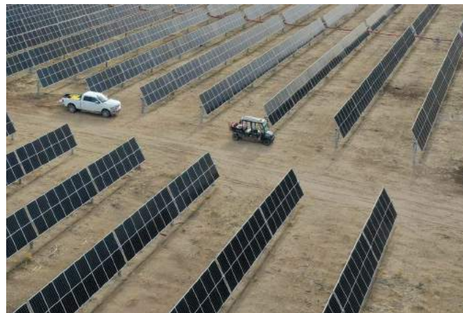
Prineville Solar Energy Center (40 MW, Solar, OR).
