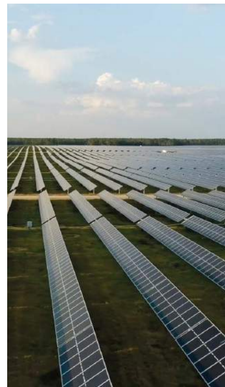
Top: The installation of bifacial solar panels at our Southern Oak Energy Center (180MW, Solar, GA). Above: Aerial view of Southern Oak Energy Center after completion.
