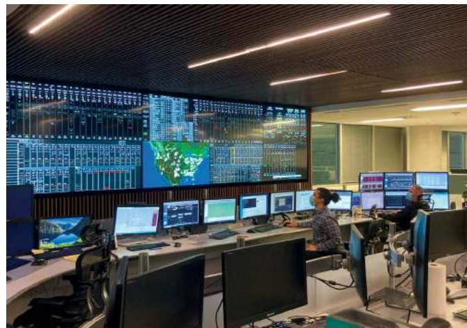
Employees working in the Invenergy Control Center (ICC) located in our Chicago headquarters.
