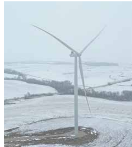
Outlaw I Wind Energy Center (96.2 MW, Wind, MO)
