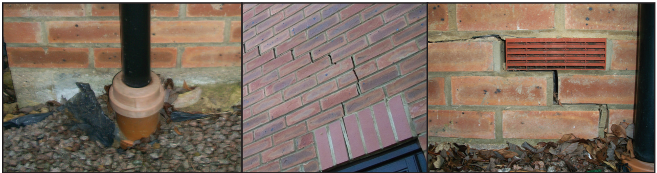
Shrinkage of clay soils due to moisture extraction from adjacent trees, LHS - 150mm reduction in ground level exposing trench blocks & drainage socket, Mid & RHS up to 15mm stepped superstructure cracking
