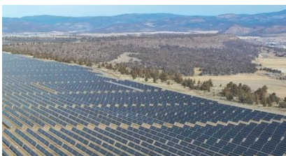
Invenergy's Prineville & Millican Solar Energy Center located in Crook County, Oregon.
